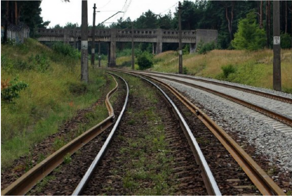
Picture 7. Buckling of the rail due to its inappropriate unload and hold in the horizontal curve (source: own archive)
