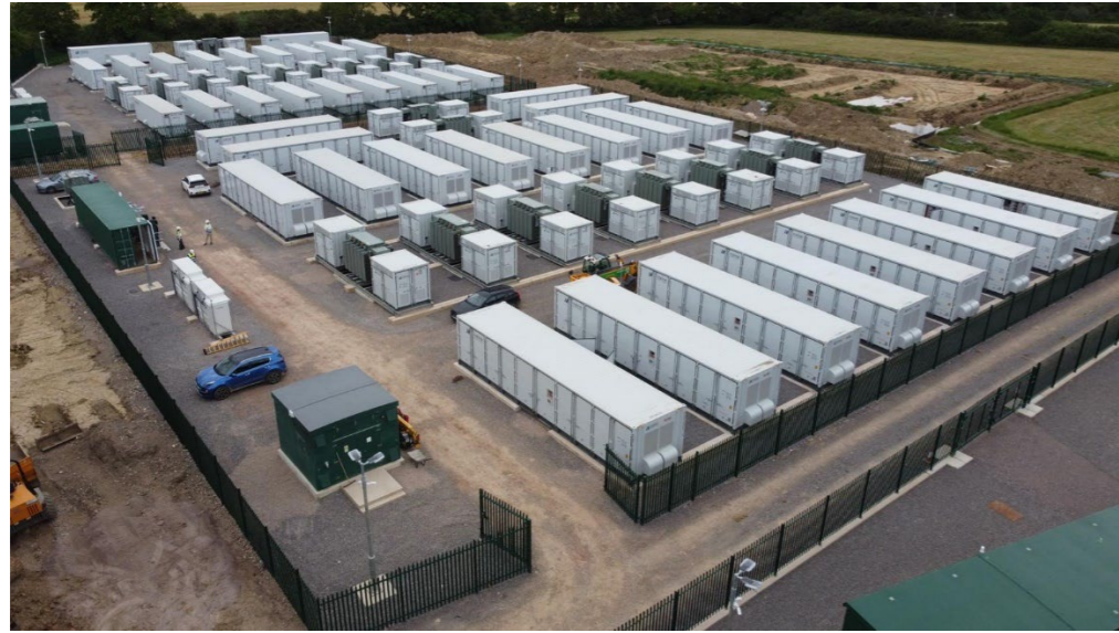
Image 1.3 Photograph of Minety battery storage; an example of a 100MW site
