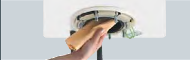
Inexpensive servicing – Servicing personnel can clean the storage heater reservoir simply and conveniently through the large flange opening.
