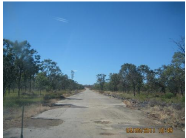
Figure 8 Jatbula Road (Mine Access Road) cross section – localised poor pavement condition, view to north
