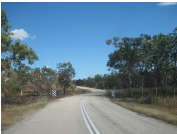
Figure 5 Edith Falls Road typical two-lane two-way cross section, creek crossing, view to west
