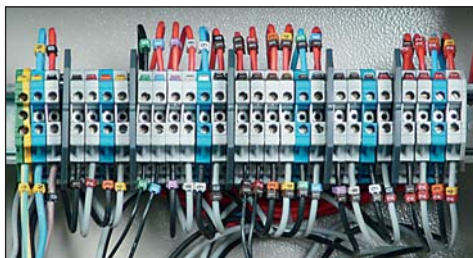
Terminal block built into the cabinet
