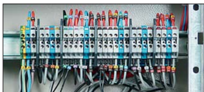
Terminal block built into the cabinet
