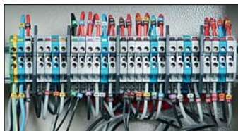
Terminal block built into the cabinet
