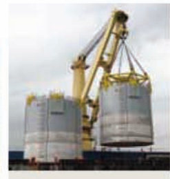
600T Concrete Caissons Fabrication For Gordon Project - Barrow Island LNG Plant, Australia
