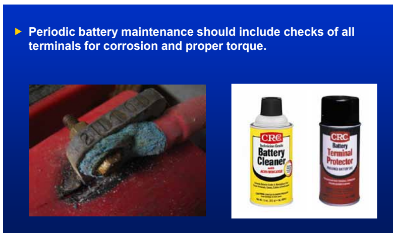
Figure 115. Periodic battery maintenance should include checks of all terminals for corrosion and proper torque.
