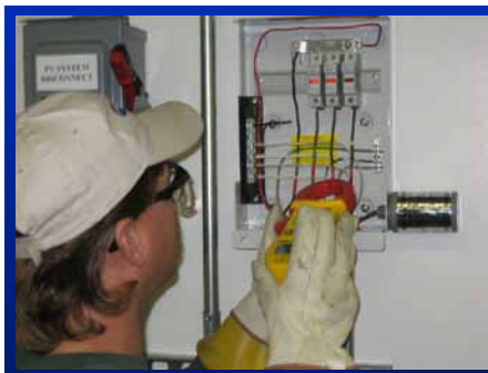
Figure 111. Operating parameters in PV systems are measured to verify expected performance.
