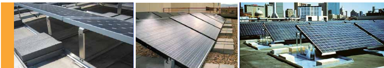
Figure 22. Self-ballasted PV arrays are a type of rack mount that relies on the weight of the PV modules, support structure and additional ballast material to secure the array.
