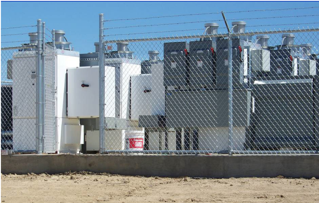
Figure 74. Utility-scale inverters use higher DC input and AC output voltages to reduce losses, and the size and costs of the conductors and switchgear required.
