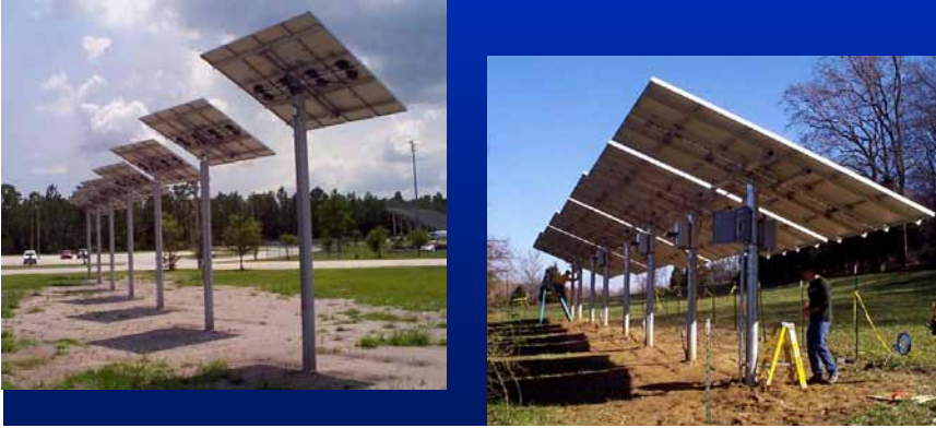
Figure 23. Pole-mounted arrays use either fixed, adjustable, or sun-tracking arrays installed on a rigid metal pipe.
