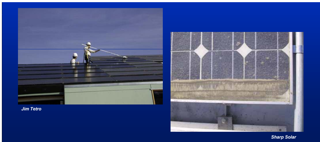
Figure 114. Cleaning soiled PV arrays is a common maintenance need.
