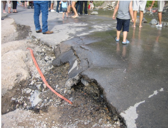
Water erosion undercuts an asphalt trail surface, posing a safety issue for trail users and costly maintenance repairs.
