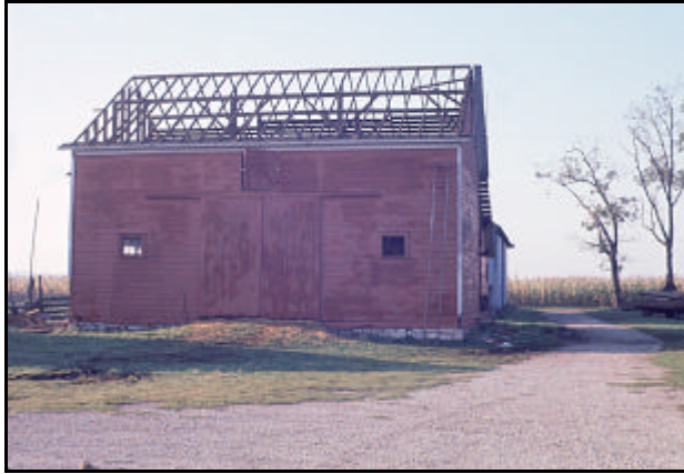
Figure 7.59 William I. Johnston's barn giving way to a modern building. Summer through Winter, 1962.
