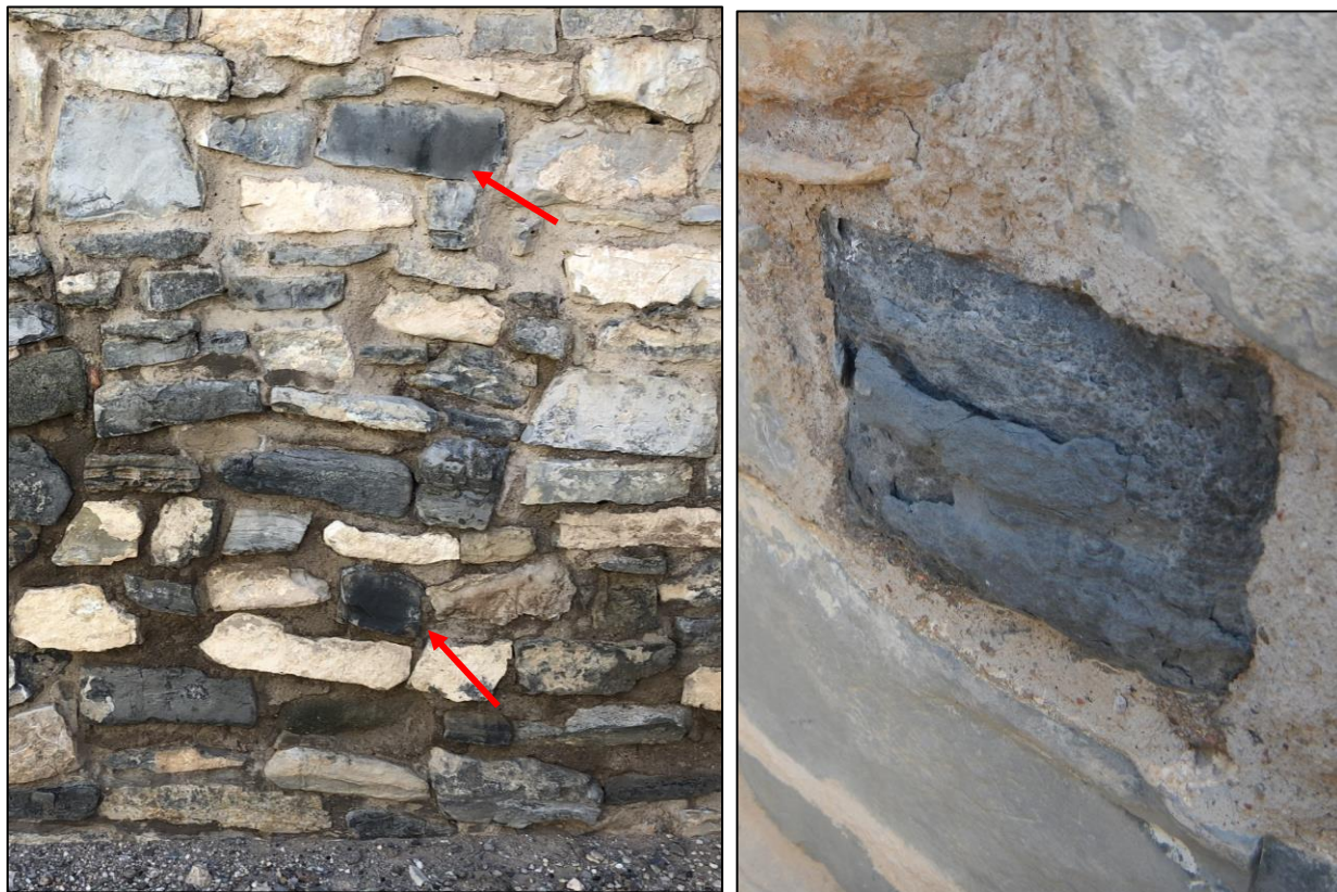
Figure 63. Evidence of past seepage events can be seen in the darker, oily appearance of rocks in the Gran Quivira church walls (left, red arrows). Rocks that experience seepage appear more likely to flake or crumble, as seen on the right (GSS photos).
