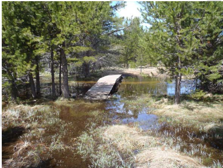
Photo 1: Unauthorized Bridge over Main Branch Angora Creek does not span the entire channel and is not constructed to DPR standards
