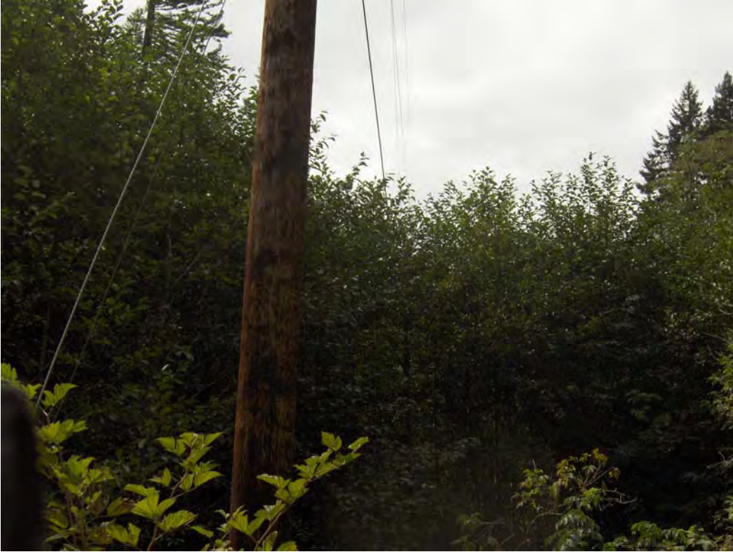
Picture 4. Picture of typical vegetation growth under and adjacent to transmission power lines along Hamilton Road on Redwood State Park property.
