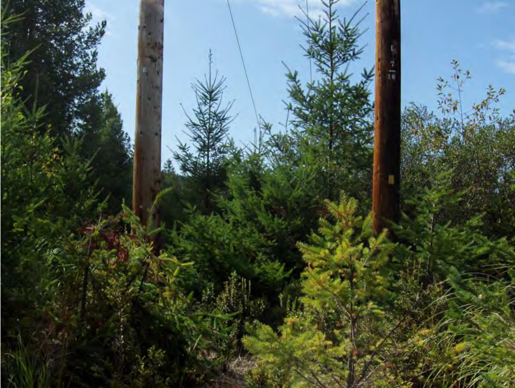
Picture 9. “H” structure poles requiring 25 feet of radial vegetation clearance off West Branch Road park spur.
