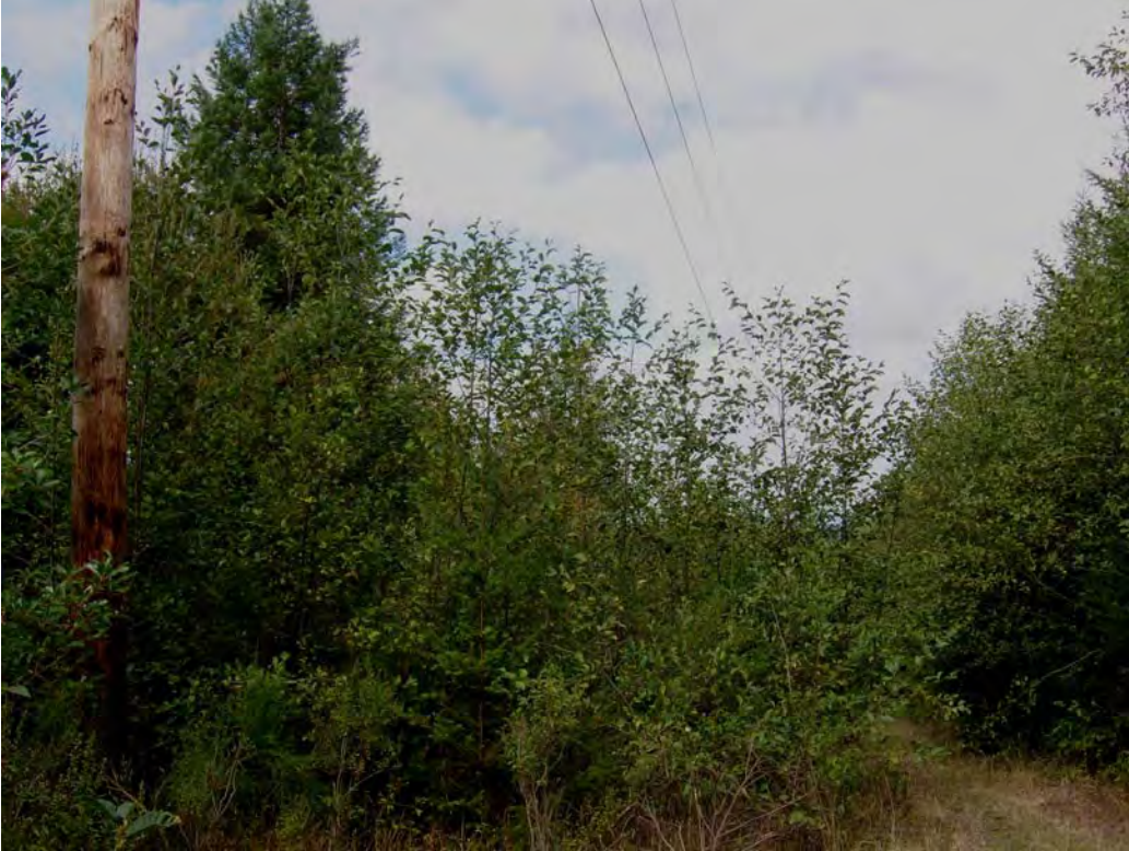
Picture 5. Picture of vegetation growth under facilities near Boy Scout Road on Redwood State Park property.
