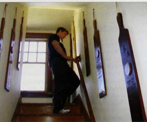
Below: The stairway at the Kappa Lambda house is now safer and more attractive.
