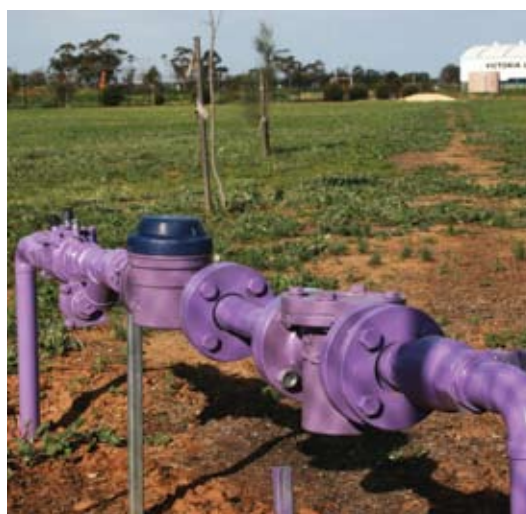
Figure 16 Recycled water meter assembly with purple to identify it contains recycled water.
