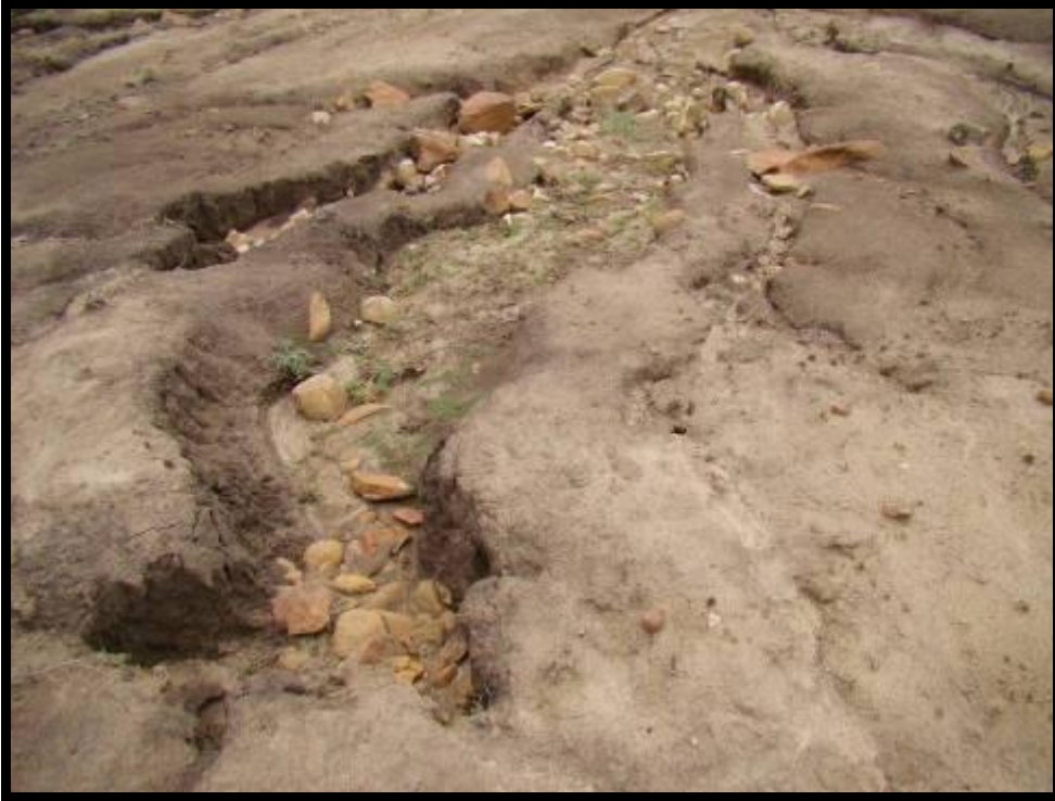
Figure 15. Extensive surface, rill and gully erosion occurs adjacent to the proposed road alignments.
