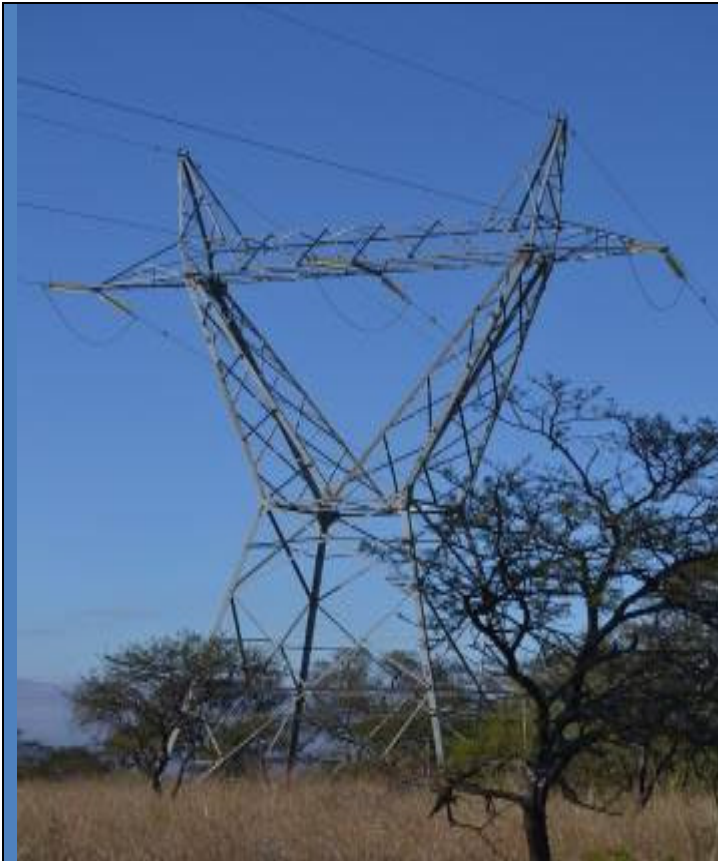
Figure 24: Lattice tower of the existing 132kv line in the Kudu Ranch Reserve
