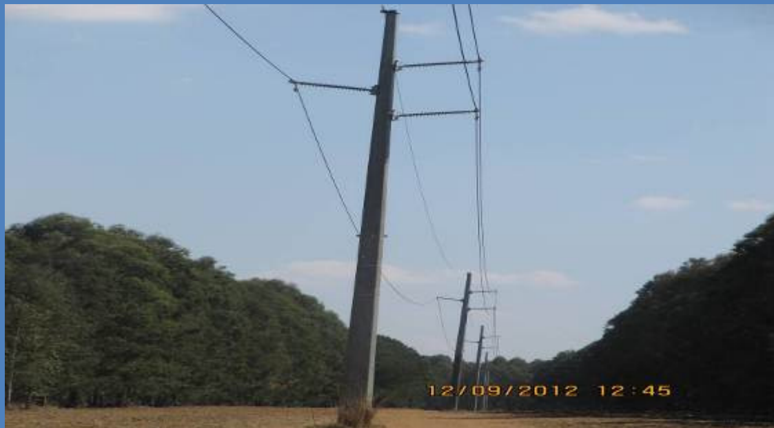
Figure 3: 132 kV steel monopole structure.
