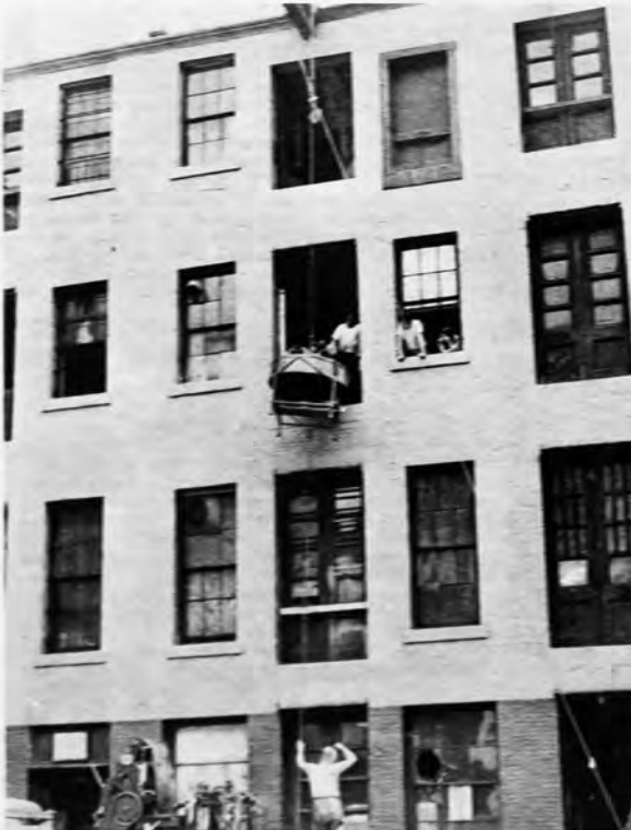
The whirler, which sensitizes offset plates, is about to be pulled into the new plant. The offset press, still on the truck, was almost at that height when it ran into trouble. The hoisting beam that caused so many hearts to jump into as many throats for a nerve-racking ten minutes is seen on the roof.
