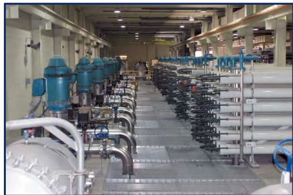
Reverse Osmosis Train
