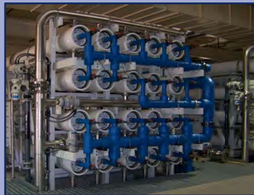
Reverse Osmosis Train
