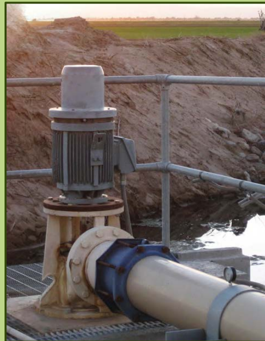
Seepage interception pump Used by permission of IID
