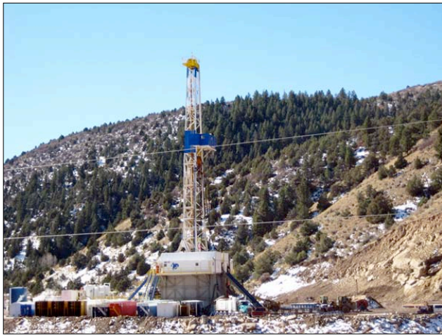
A gas drilling rig located along Piceance Creek in Colorado. The current oil and gas boom in and around the Piceance Basin has had a powerful impact on nearby communities in Garfield, Mesa, and Rio Blanco Counties. Credit: Jason L. Hanson (Oct 2007)
