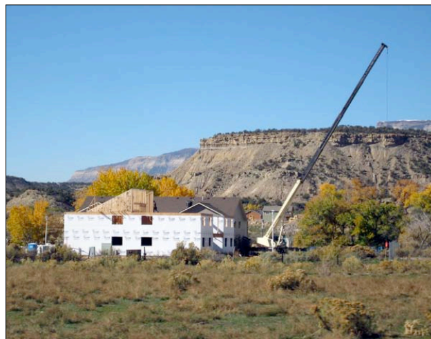
A new building goes up on the outskirts of Rifle, Colorado. The influx of people arriving to work on the area's oil and gas operations has left housing in short supply in towns like Rifle. An oil shale boom overlapping with the current oil and gas boom could exacerbate the shortage. Credit: Jason L. Hanson (Oct 2007)
