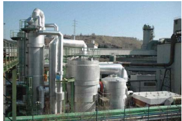
Figure 3—CORE™ installation processing gas up to 21 vol% SO 2 and operating since 2009
