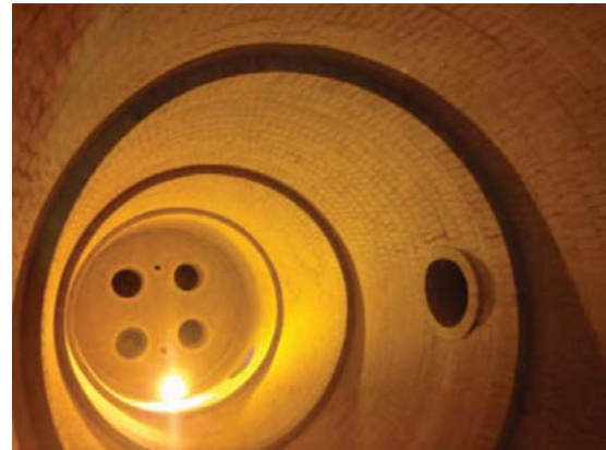
Figure 5—Sulphur furnace internals
