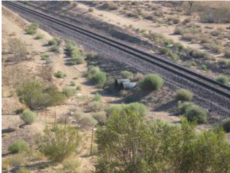
PHOTO 7. Looking northeast at BNSF Railroad at culverts that provide drainage for the tracks.
