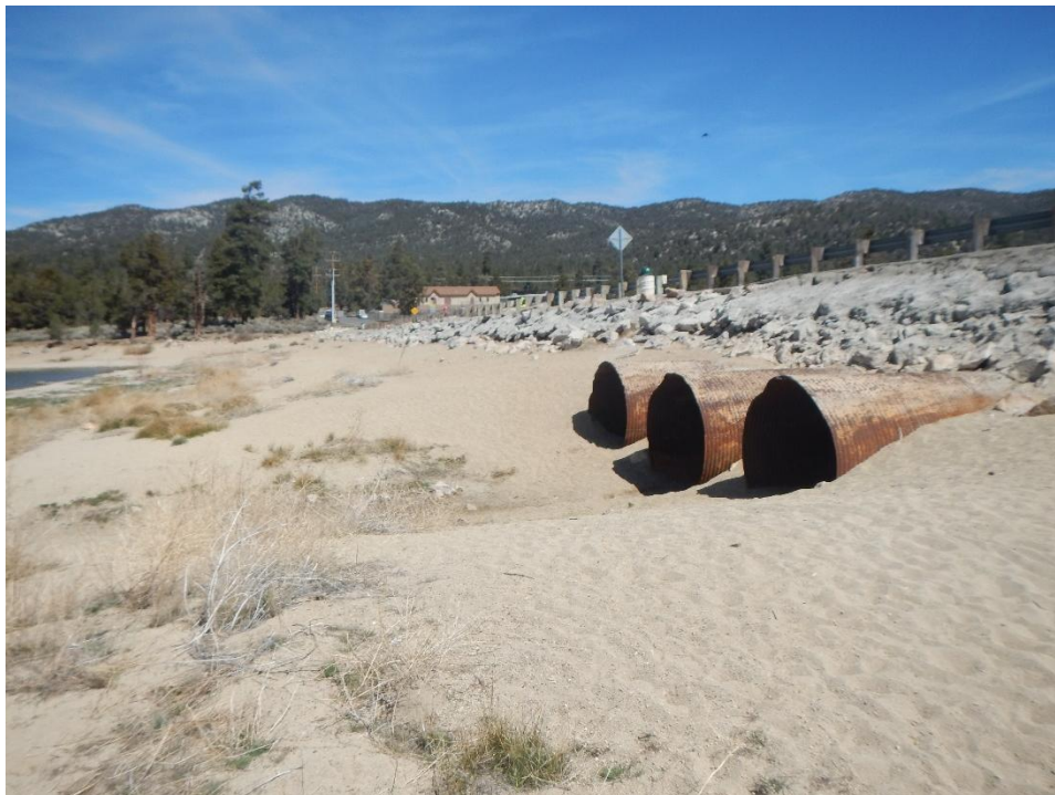
Photo 4: Big Bear Lake bank and culverts on the western border of Stanfield Cutoff, looking northeast.
