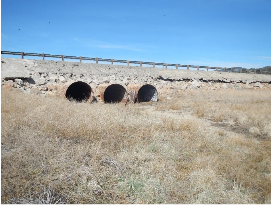
Photo 1: Big Bear Lake bank scour along the eastern border and culverts going under Stanfield Cutoff, looking northwest.
