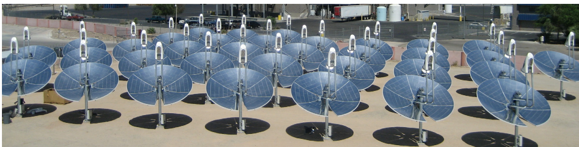
Figure 5.14 34 Infinia Corporation dish Stirling systems in operation at Yuma AZ
