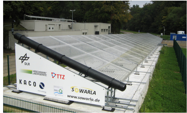
Figure 7.8 The solar photocatalytic water treatment demonstration plant in Lampoldshausen, Germany
