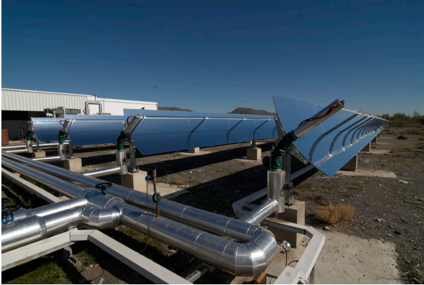
Figure 7.4 Photo of the new PTC solar field in operation at the PSA
