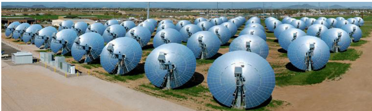
Figure 5.13 SES Maricopa 60-dish plant in operation near Phoenix, AZ
