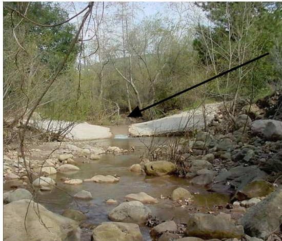
Example of old concrete crossing blocking steelhead passage
