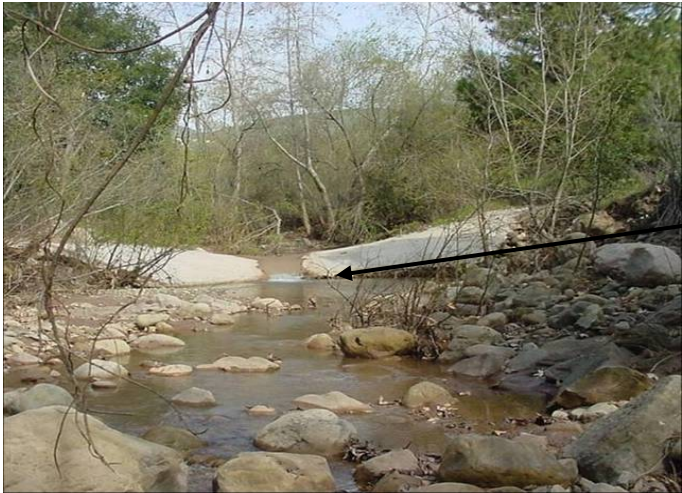
Example of old concrete crossing blocking steelhead passage
