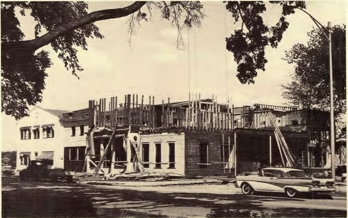
Used lumber for sale! Some of it was well used for nearly a hundred years by the time this old office building was demolished.
