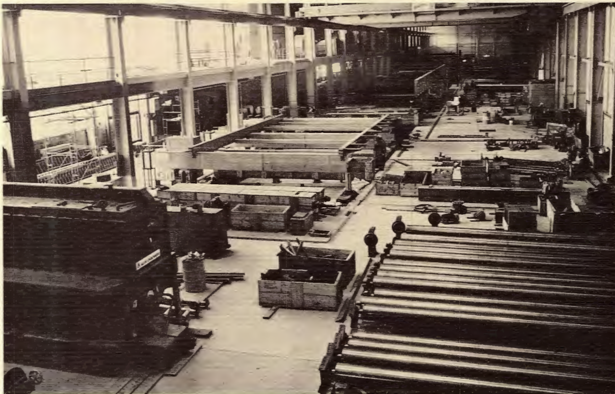
Ashdown's first paper machine is being erected in this view of the mill interior in 1967. Although a giant when built, the machine
