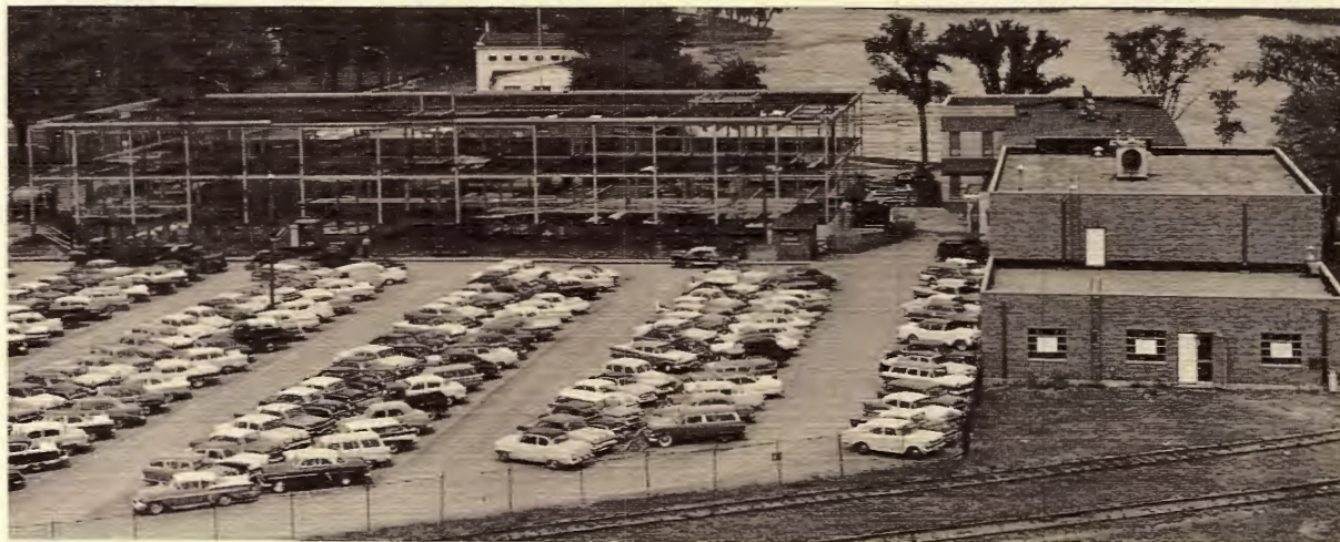
Steel framework for a new administration building for Nekoosa Papers dwarfs the old office building that it will replace. Building
