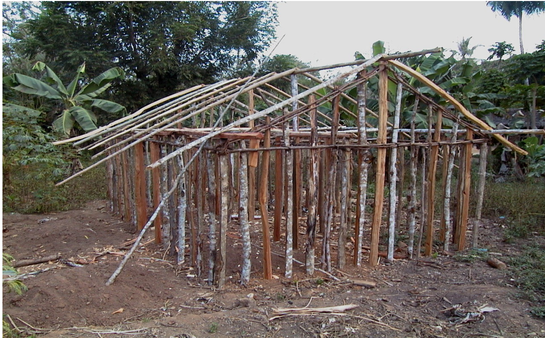
Plate 2: A local house under construction using threatened tree species around ANR. Note that poles are Allanblackia stuhlmannii while roofing materials are Cephalosphaera usambarensis
