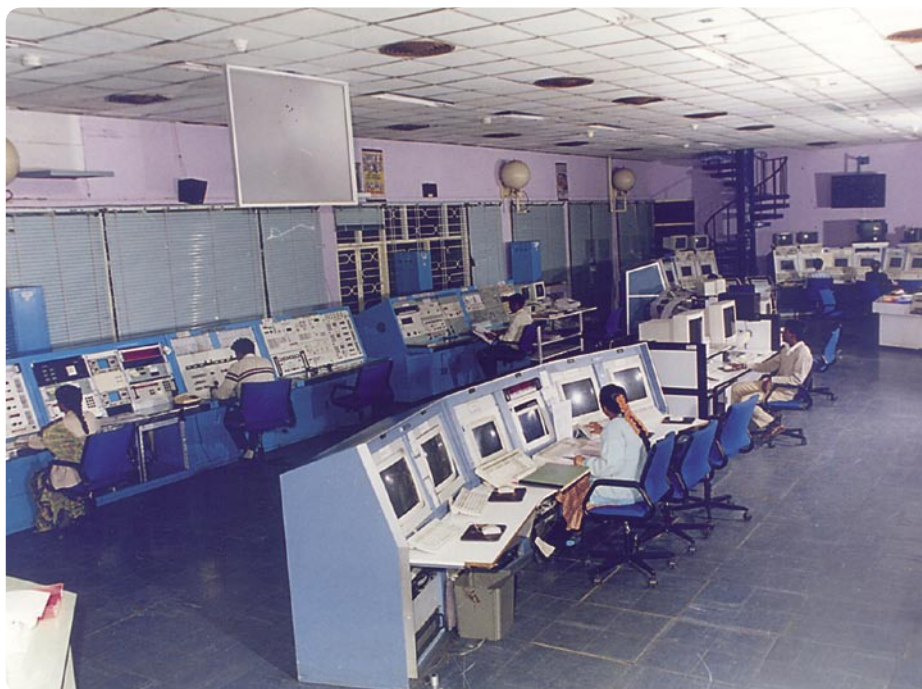
| A view into the control center for Tracking and Telemetry |
