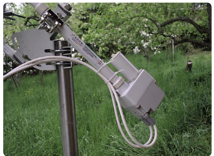
This drive motor moves the antenna support
