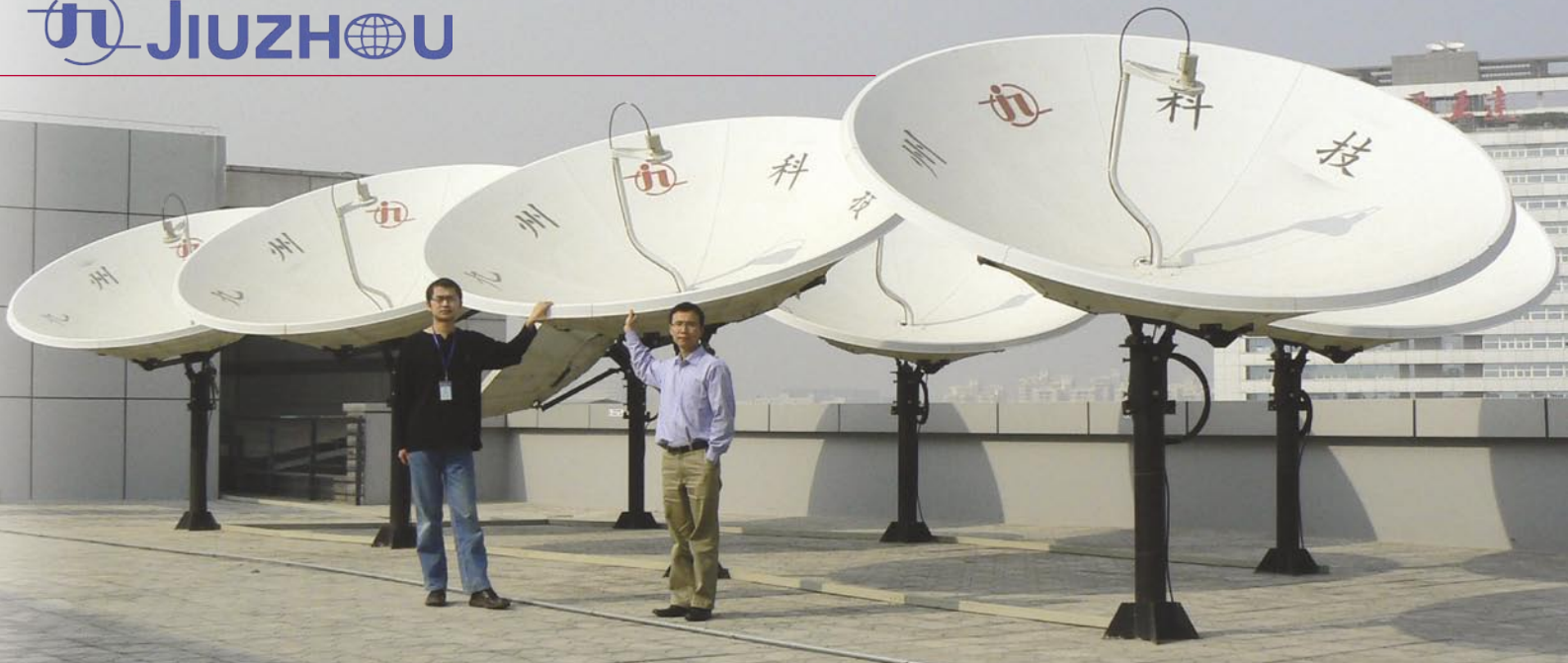
▲ On the roof of the Jiuzhou Electric building: seven dishes, naturally from their own production line, were professional erected so that the development engineers can receive all of the receivable satellites with maximum signal strength. Nung Yue, responsible for building operations, can be seen here with a developmental engineer.
