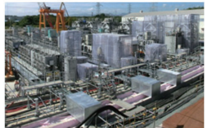
Whole view of Multiple Radio-nuclides Removal System (MRRS) (from TEPCO's website)
