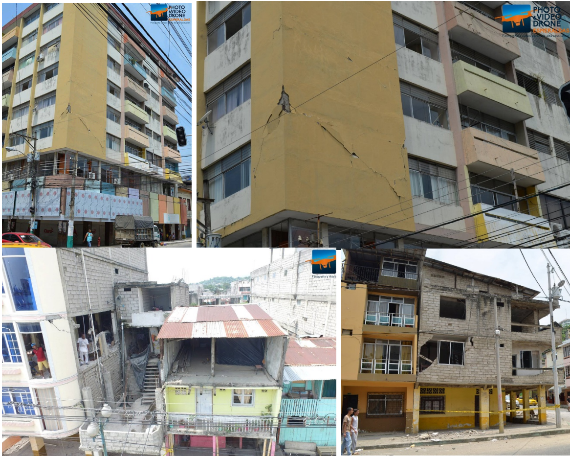
Figure 6a-d. Minor damage in the center of the city of Esmeraldas by the earthquake of Pedernales of April 16, 2016 (Mw 7.8). Upper images from left to right referring to the Bolivar and Manuela Cañizares direction. Bottom images from left to right, referring to the addresses December 6 and Piedrahita, and Ricaurte and / Colon and Eloy Alfaro. Photo courtesies: "photo & video drone Esmeraldas".
