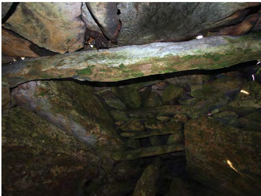
Plate 12. Interior of the roof of the Foel Fras shelter (PRN 38623), showing construction
