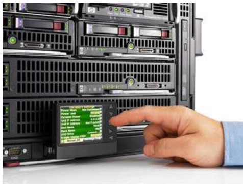
Figure 4. Insight Display on the c3000 enclosure
