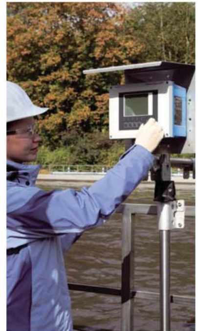
The Liquiline CM442 installed at a water treatment plant. [2]
