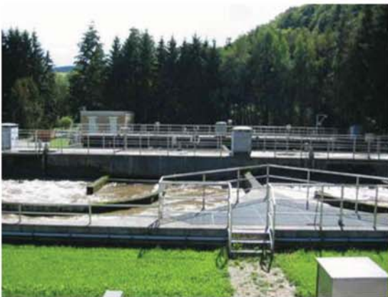
Example of a treatment plant
