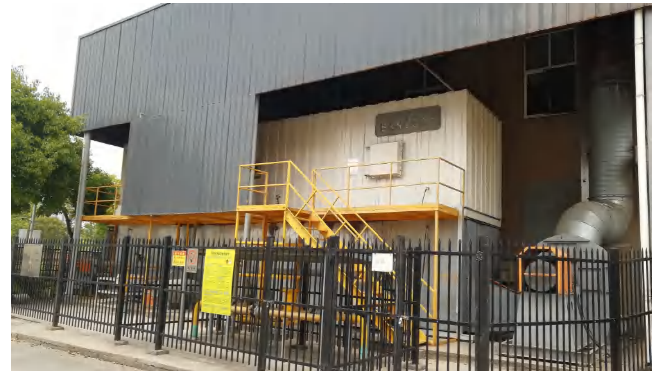
Waste gas treatment facilities
