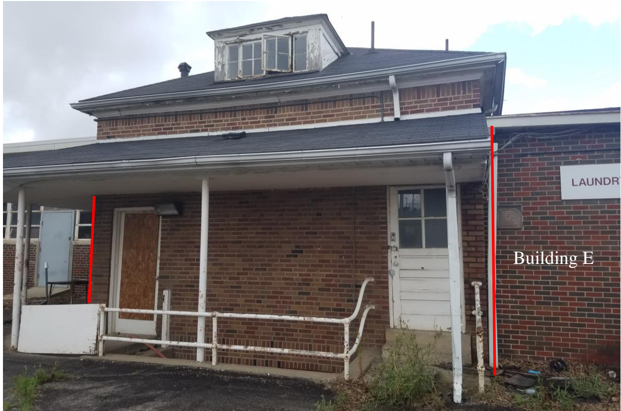
Former Airport Watch Tower (Front) Facing West with Building E additions located North and South of the Watch Tower (Photo 28)
