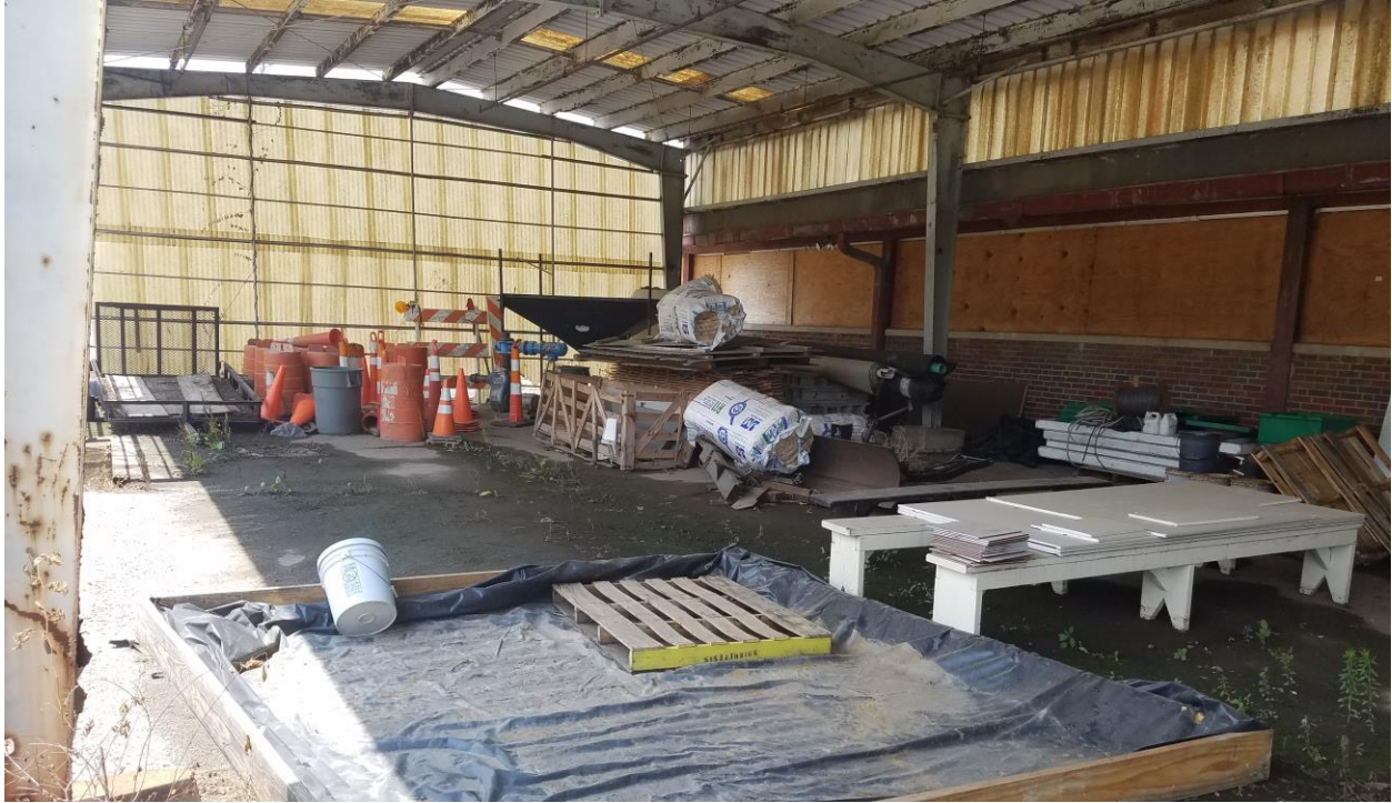
Maintenance/ Storage area located on the Southern Extent of the Subject Property (Photo 25)
