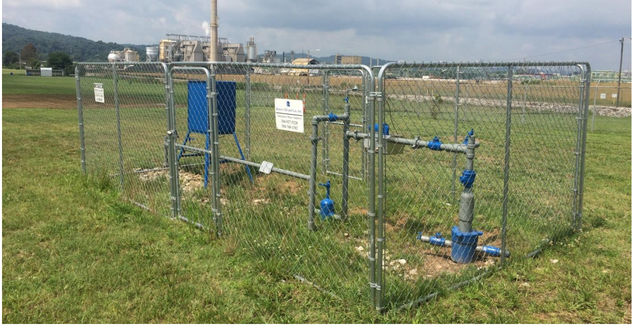
Subject Property Natural Gas Well and Regulator Facing Southwest (Photo 7)
