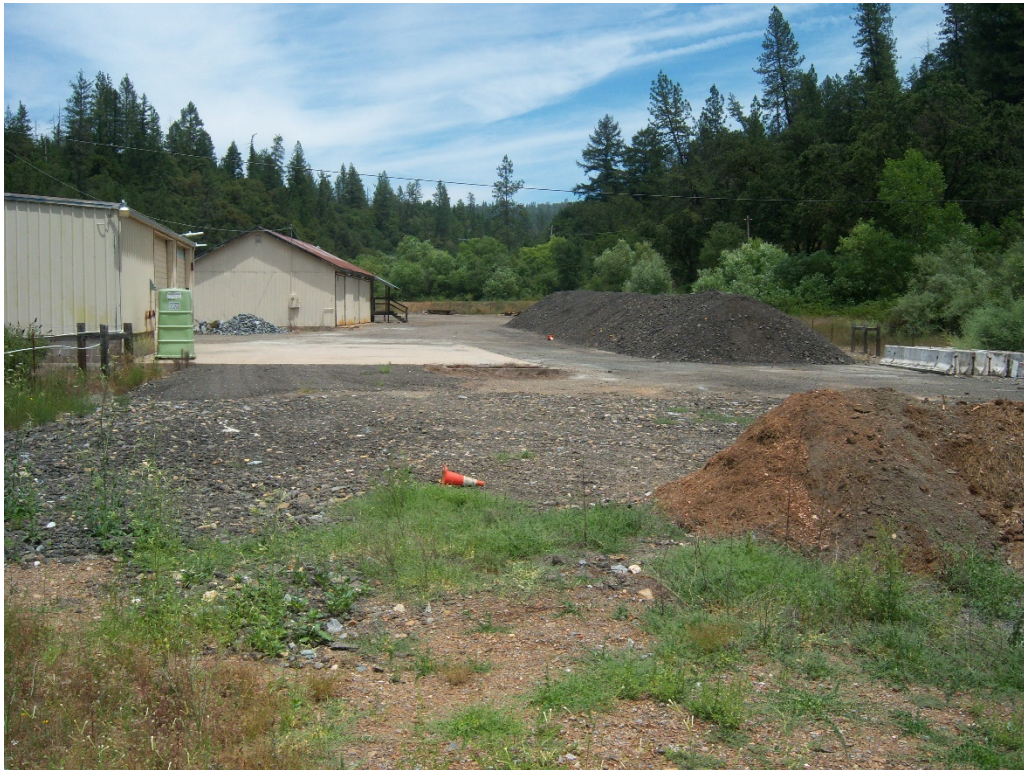
Photograph 13: Overview of two storage buildings and large pile of ground asphalt; facing northeast
