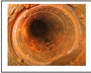
Sea Water Pipeline Without SWCI 101
