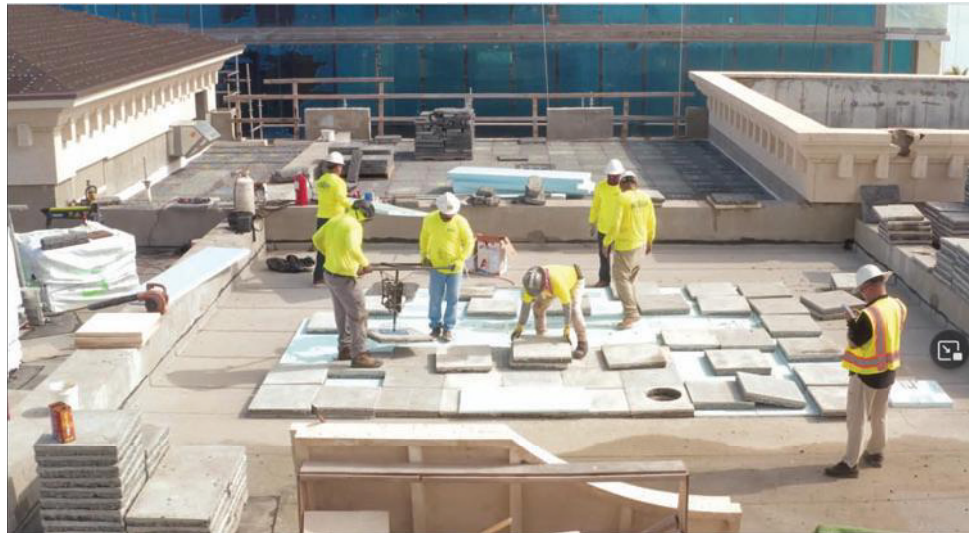
Workers installed Echo Blocks on the rooftop terrace to create a solid, flat, permeable walking surface.
