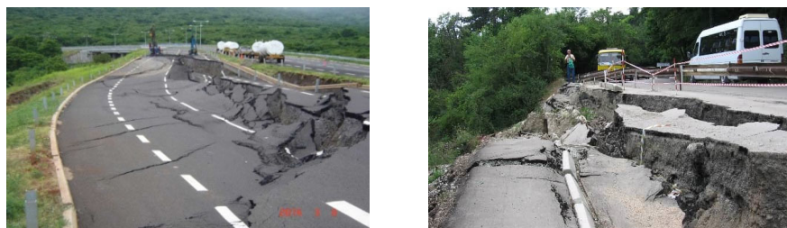
Figure 6: Typical slope failures at roadsides
