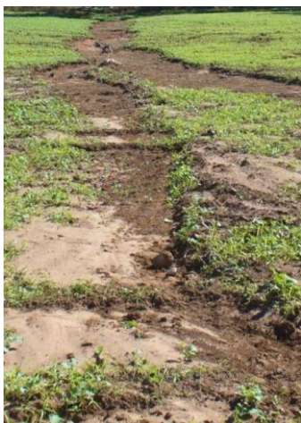
Even with ground cover, erosion can be difficult to control if the speed and direction of runoff water is not managed.
