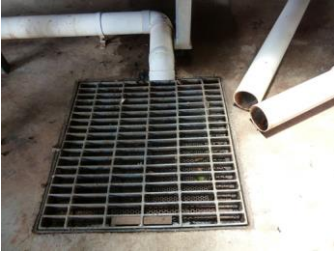
Grates in the packing shed remove banana flowers and other debris effectively from waste water.
