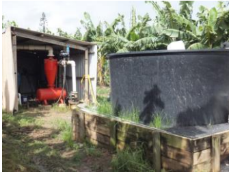
Fertigation is an efficient way to apply fertiliser.
