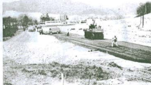
The Route 2 project demonstrates the versatility of bottom ashes when quality control and performance engineering are emphasized.
