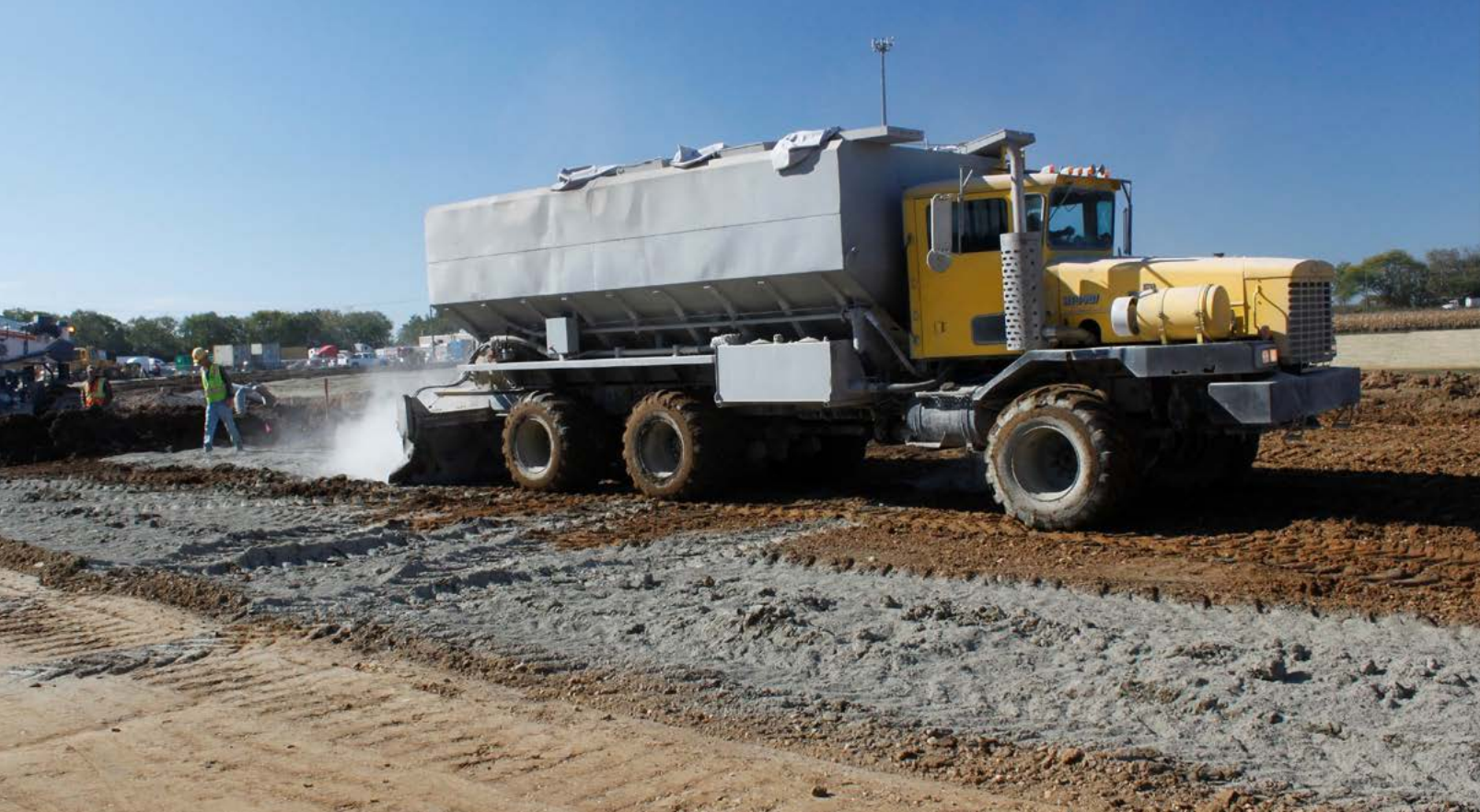
This building pad in Channahon, Illinois, uses a 50:50 blend of Class C fly ash and Type 1 cement.
