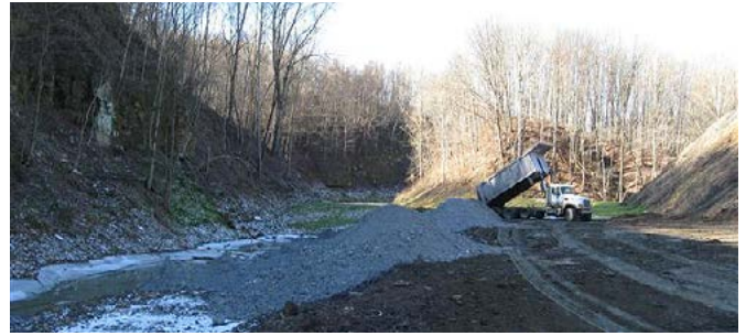
(4) First batch of sFGD in January 2012.
