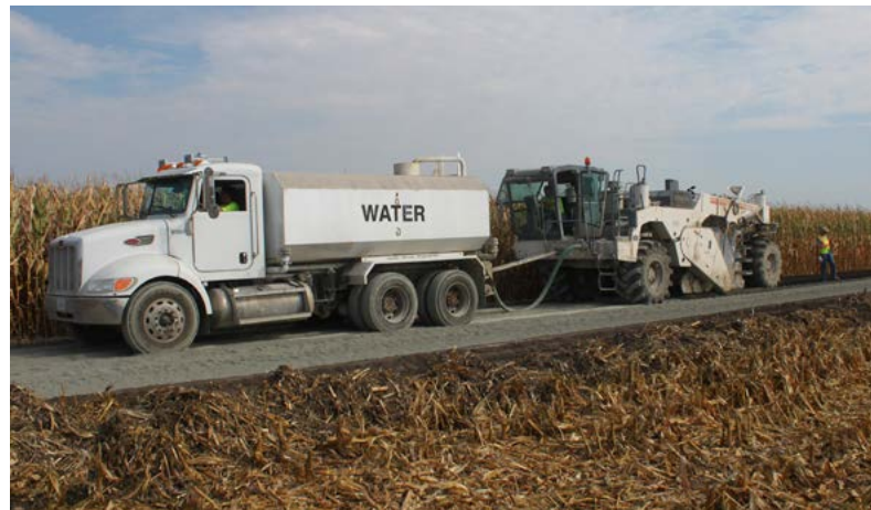
Subgrade modification of an access road at Invenegy's Bishop Hill Wind Center Phase 3 Windfarm, in Woodhull, Illinois.
