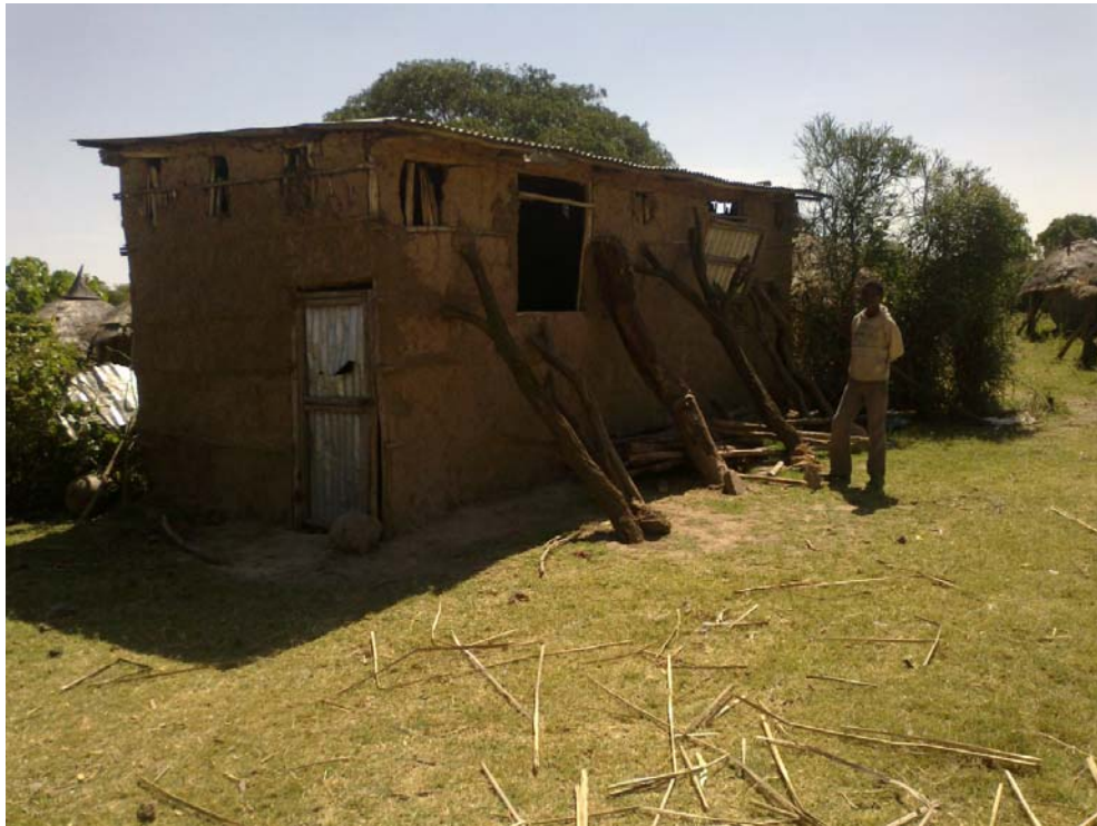
Plate 2. Termite infested houses supported by poles.
