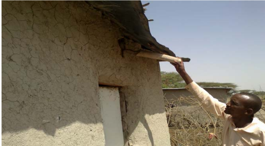
Plate 1. A roof supporting timber completely cut by termites.
