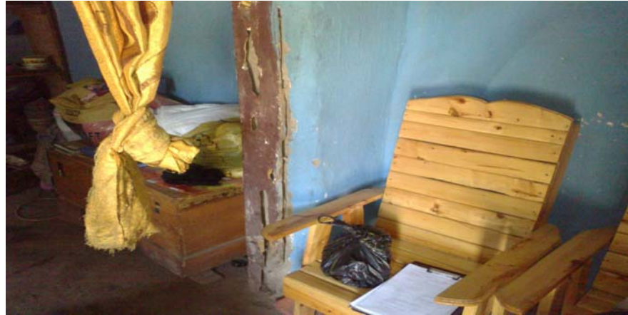
Plate 3. Severely damaged door frame.
