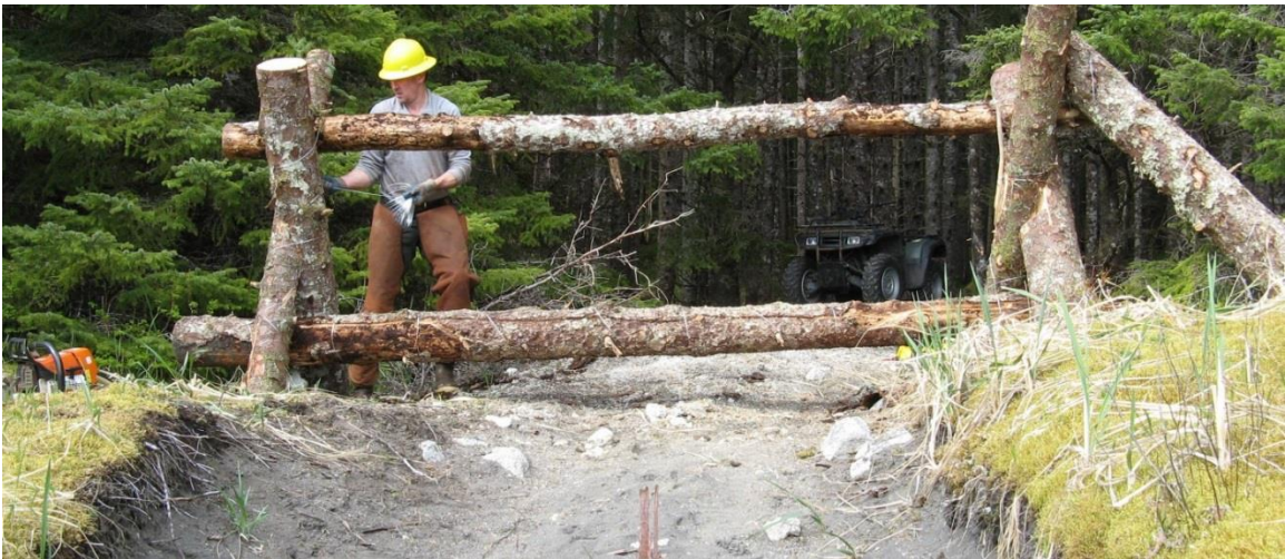
Figure 7. Barriers to prevent access to the closed portion of North Beach were constructed in May of 2013. This trail was closed because access to the lower beach was unsafe due to erosion. Photo by Brad Kriekhaus, USFS.
