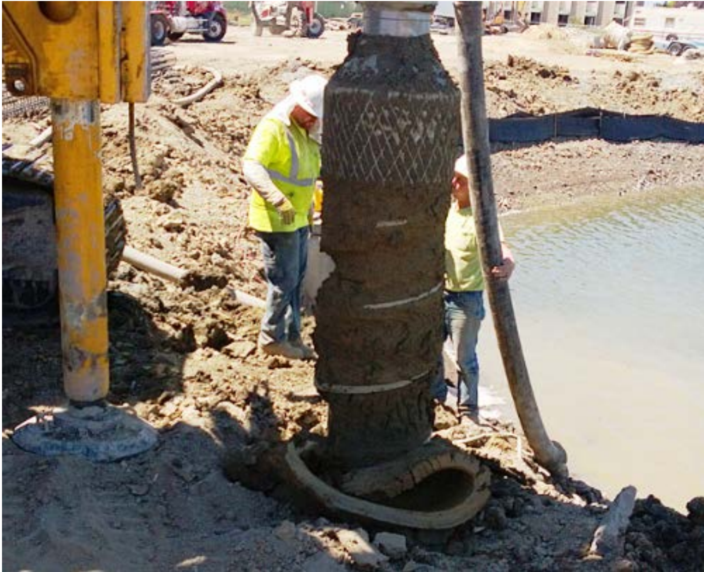
Figure 112. Photograph of a DDC auger bit and grout injection line (being held by worker) (Source: image courtesy of Jeremy Zorne)
