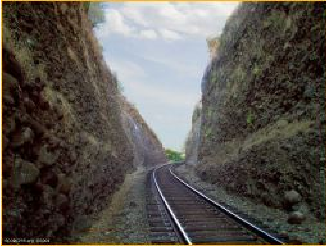
Figure 8-A. Midway in Bloomer Cut looking east ca. 2015. Note that the cut is not terraced, and the walls are near vertical. (Courtesy of Bruce C. Cooper, CPRR.org ).
