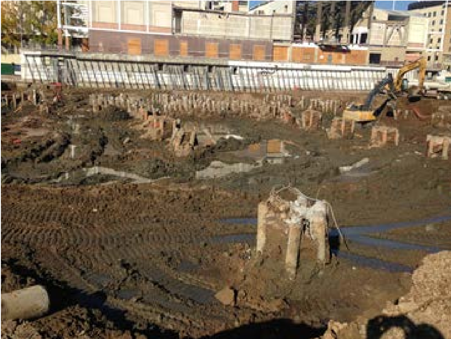
Figure 114. Photograph of soft and wet ground conditions and stick up of a few driven piles that supported the former downtown plaza development (Source: image courtesy of Jeremy Zorne).
