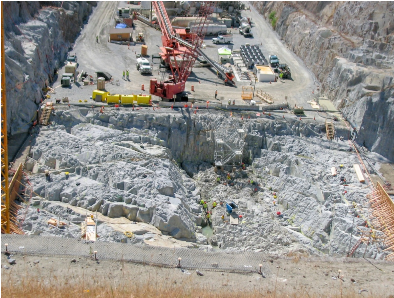
Figure 125. Completed foundation excavation of the Folsom Auxiliary Spillway Control Structure looking downstream. The excavation achieved a slightly weathered to fresh granitic rock surface. The over-excavation in the center of the excavation was to remove poor rock associated with two parallel shear zones trending up and downstream. Workers are performing final cleanup prior to initial concrete placement. (Source: image courtesy of William A. Fraser).
