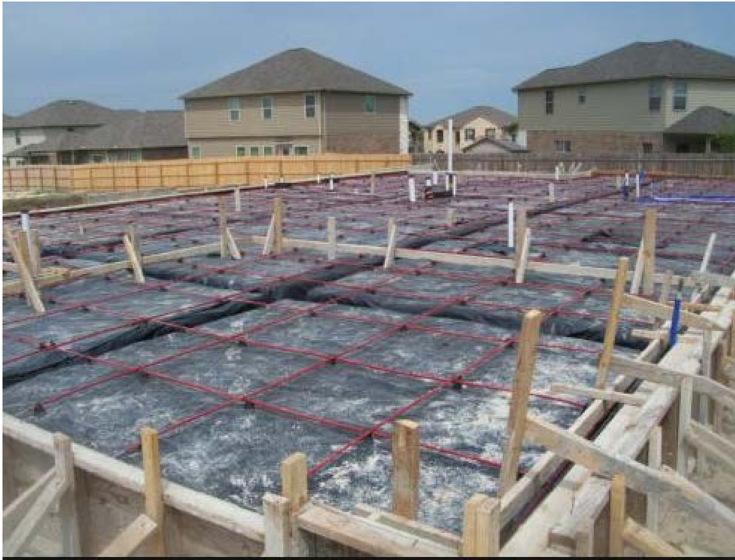
Figure 110. Photograph of a typical post-tensioned slab foundation (Source: image courtesy of Jeremy Zorne).
