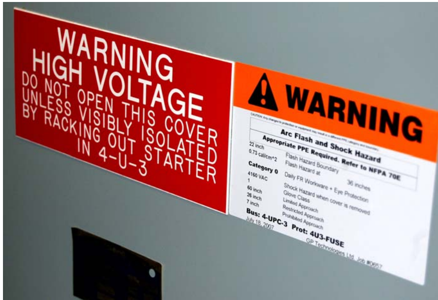
Photo 5.5: Warning labels on outside of door to power factor capacitor cell 4-U-3. The labeling is common to all power factor capacitor cells in 4-ESB-1.
