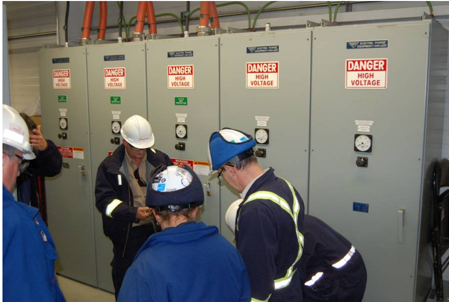
Photo 5.3: Power factor capacitor cells.
