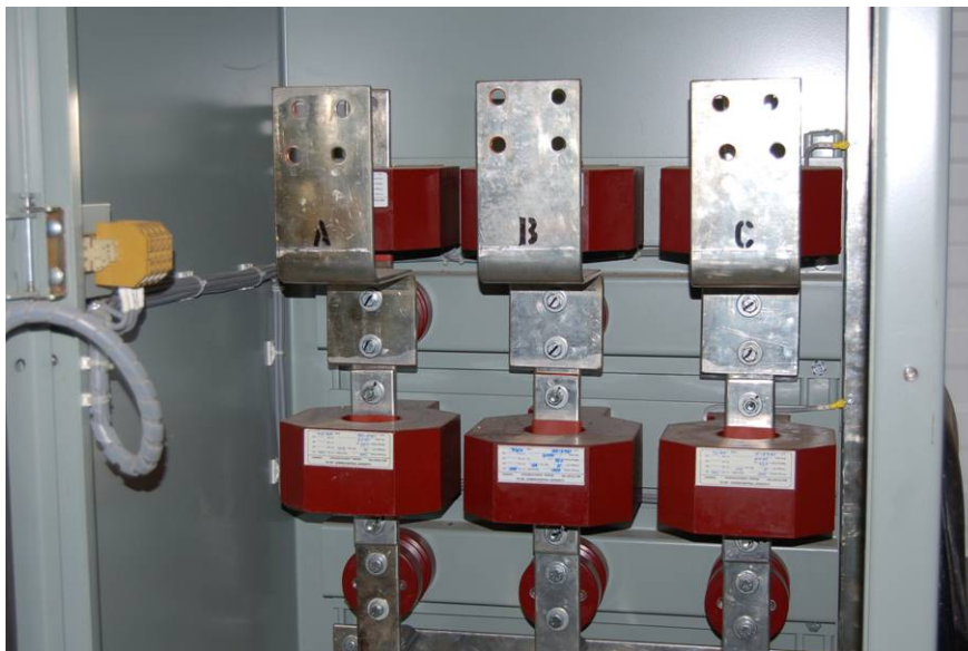
Photo 5.4: inside of power factor capacitor cell 4-U-2.
