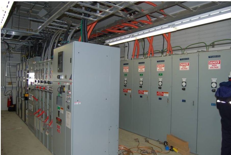
Photo 5.2: Unit starters and power factor capacitor cells.
