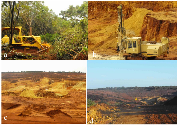
Figure 3. a) Original forest cover clearing, b) Drilling works by using heavy machines, c) Large scale mining area for limestone, d) Newly established mining area
