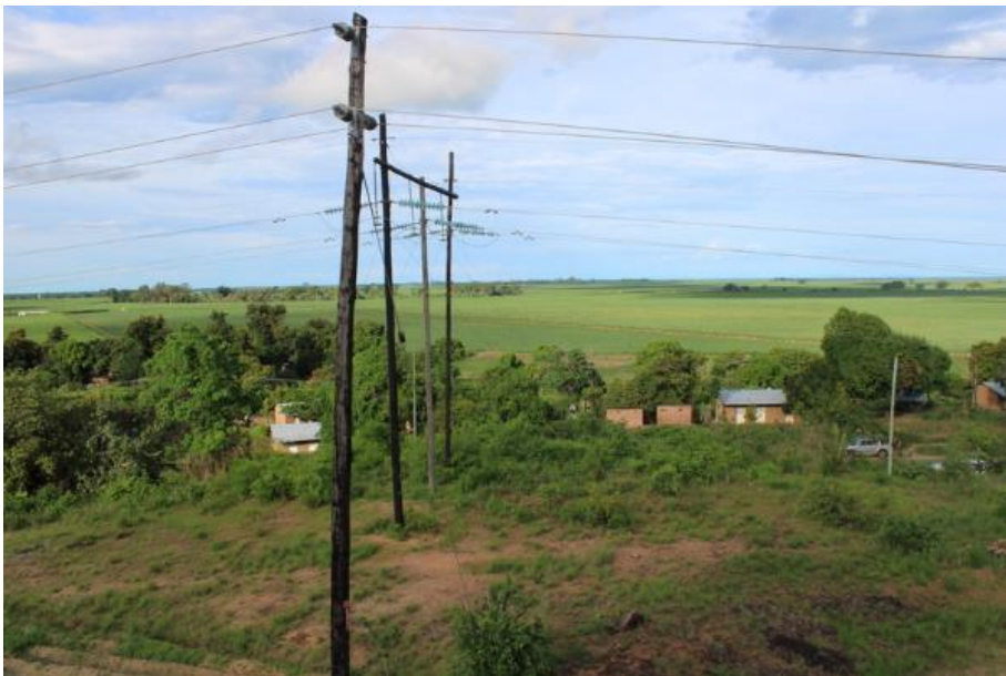
Figure 7.11 Overhead lines transverse through the site
