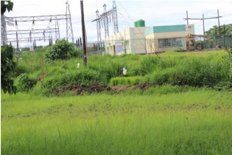
Figure 7.10 Existing ESCOM substation
