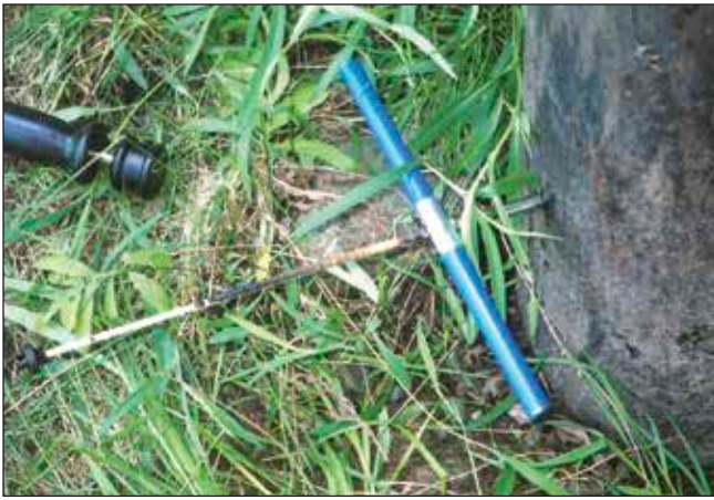
Figure 5.8 —An increment core can be used to conduct inspections of timber bridge elements. This image shows an extracted core from an in-service timber pile ready for examination.
