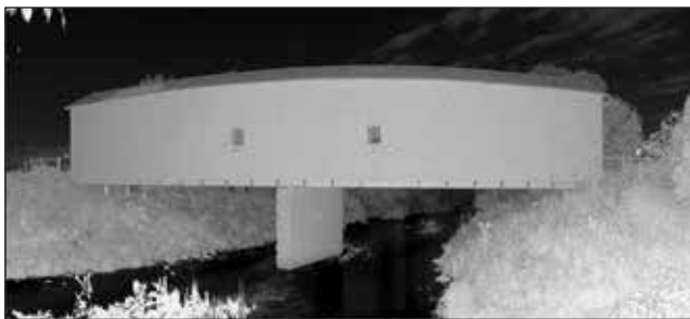
Figure 13.30—Scalar image of the outside of the Zumbrota Bridge created from a single exterior scan processed with Faro Scene software.
