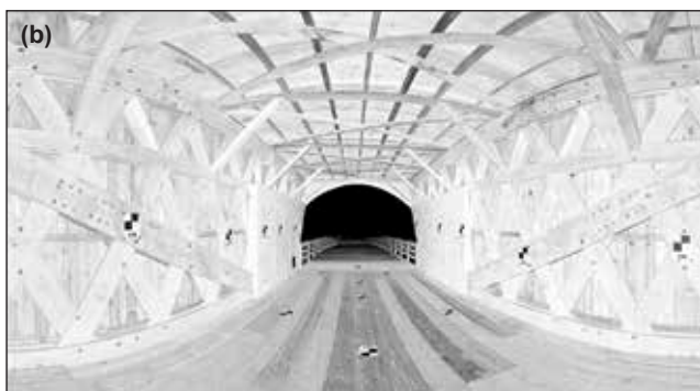
Figure 13.24—Planar views of a single laser scan of the Roseman Bridge (NRR).
