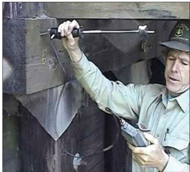
Figure 5.7—A pin-style moisture meter is used to determine moisture content of timber elements.
