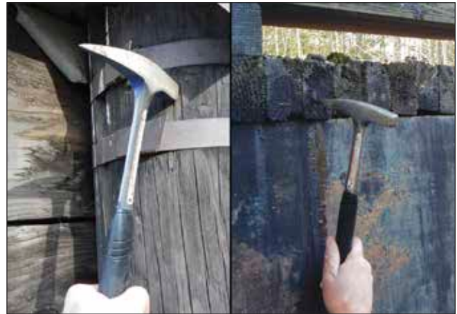
Figure 5.1—A hammer pick is an effective tool for initial assessments of timber bridge elements.
