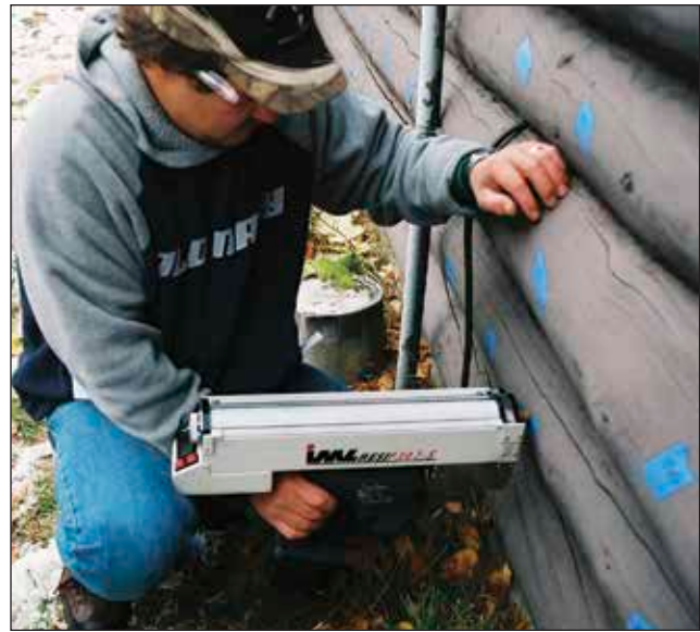
Figure 5.9 —A resistance microdrill used for inspection of a historic Civilian Conservation Corps log cabin.
