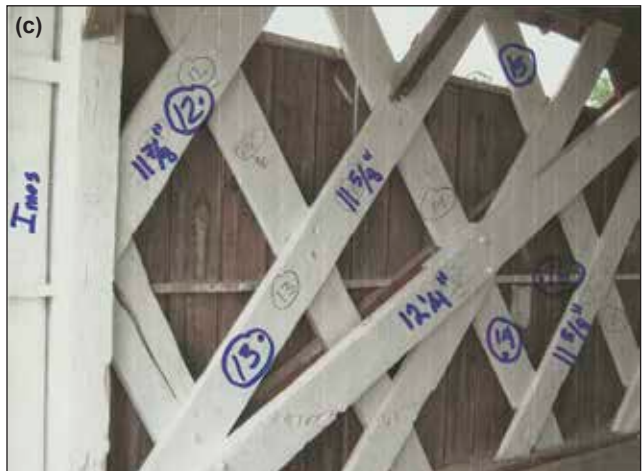
Figure 13.39—Locations on the Imes Bridge where comparison measurements were taken using traditional tape measures and extracted from the digital point clouds created from the laser scanning process.
