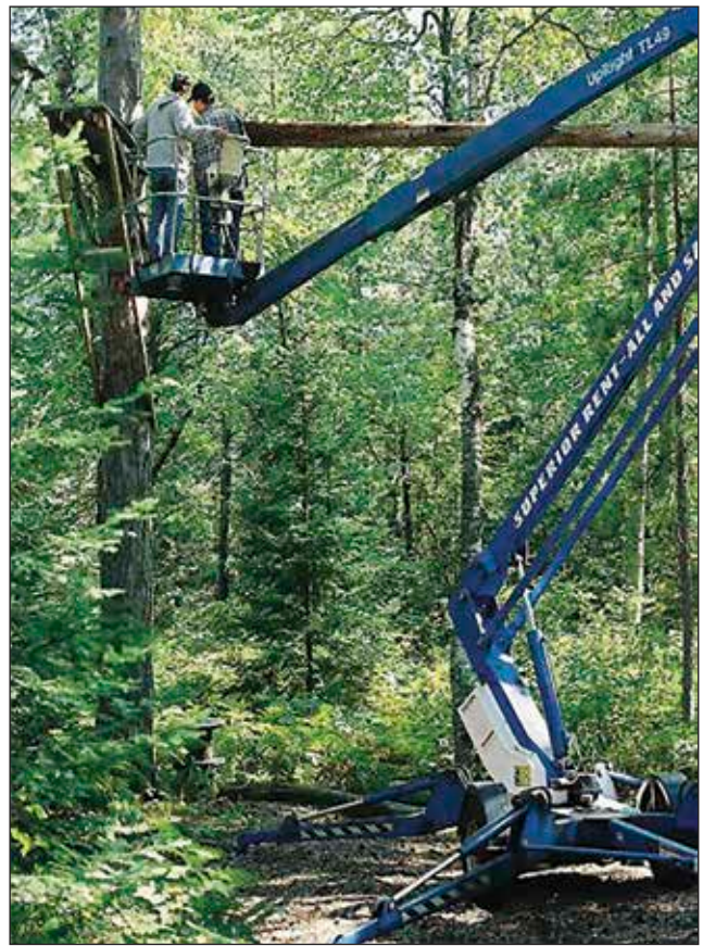
Figure 7.8—Case study at the U.S. Forest Service Nesbit Lake Camp, Sidnaw, Michigan—Visual and nondestructive evaluation of red pines supporting a ropes course.
