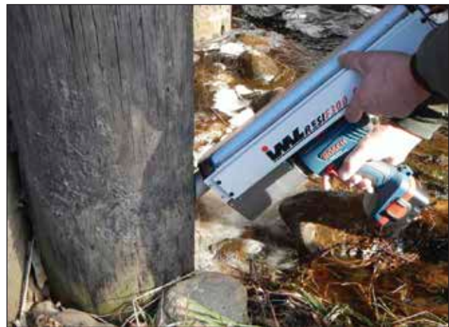
Figure 5.11 —Drilling can take place at an angle to assess the area below ground line.
