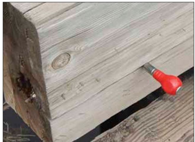
Figure 5.2—An awl is used to assess depth and presence of decay in a horizontal split.
