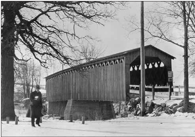
Figure 13.1—Photograph of the Cedarburg Covered Bridge (Cedarburg, Wisconsin), circa 1934. From the Library of Congress.
