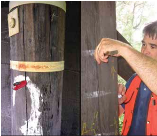
Figure 5.3—Probes are used to assess depth of cracks, checks, and through splits in timber bridge elements.
