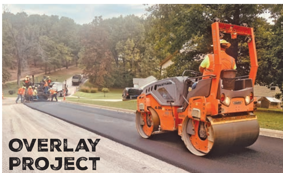
Workers with Capital have started the overlay projects throughout the city of Harrison by repaving the streets at Country Circle. The surface is being repaved with two inches of asphalt. Selected streets on the overlay project list include Lakeshore Drive, East Bower Avenue (Main to Walnut), West Bower Avenue (Main to Maple), Highland (Capps to Stephenson), North Industrial Park Road (Airport Road to Johnson Road), Johnson Road (North Industrial Park Road to Industrial Park Road), South Sycamore (South Walnut to East Rogers), Bunker Road (Cottonwood Road to Harness), and First National Bank Road. CONTRIBUTED PHOTO/LEE H. DUNLAP
