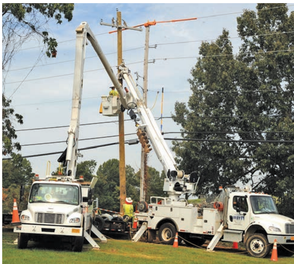
Entergy subcontractor IRBY Construction has started upgrading the power line work on Capps Road. Customer Service Manager Mark Martin said "The upgrading will be from Goblin Drive, west on Capps to 397, and then north on 397 to 43. This will allow for growth and improve reliability on this circuit. The project should be completed by year end excluding any unforeseen issues or storms. Entergy continues to upgrade and improve our facilities." CONTRIBUTED PHOTO/LEE H. DUNLAP
